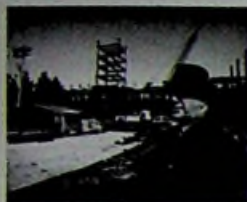
President R.F. Thompson views construction of the science building that will be named for him.
