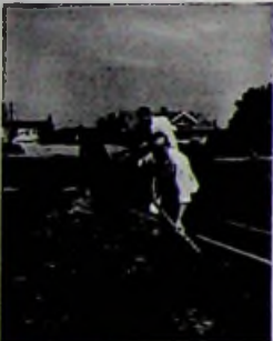
Dean John Regester helps students dig trenches for water lines on Campus Day, May 1949.
